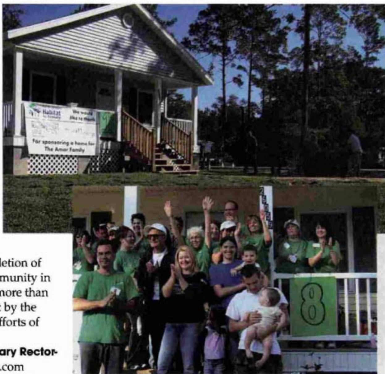
With the recent completion of 10 homes, Hairdressers Unlocking Hope has completed the first phase of its goal to construct 20 houses.
